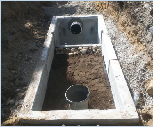
Photograph 6: Roosevelt Avenue filtering catch basin 2.
