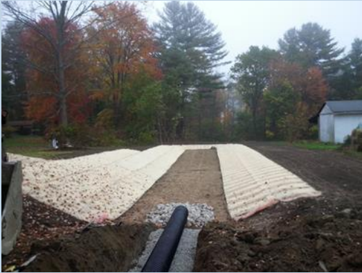
Photograph 2: Bioretention system at lower Horne Street
