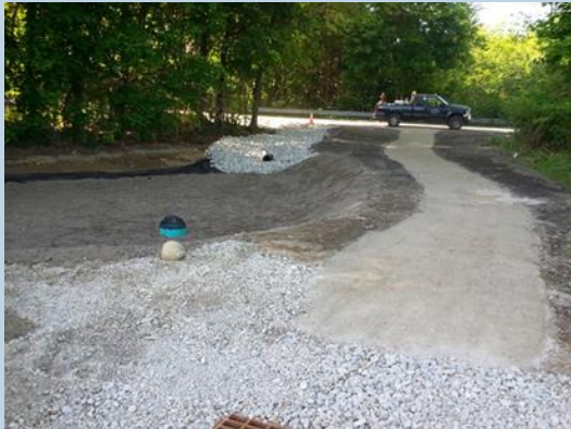
Photograph 1: Bioretention system at Roosevelt Avenue
