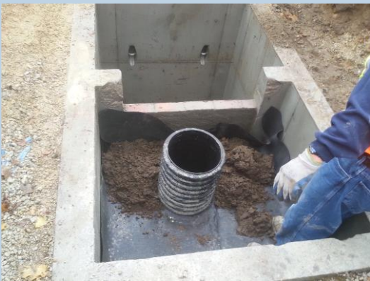
Photograph 3: Roosevelt Avenue filtering catch basin 1.
