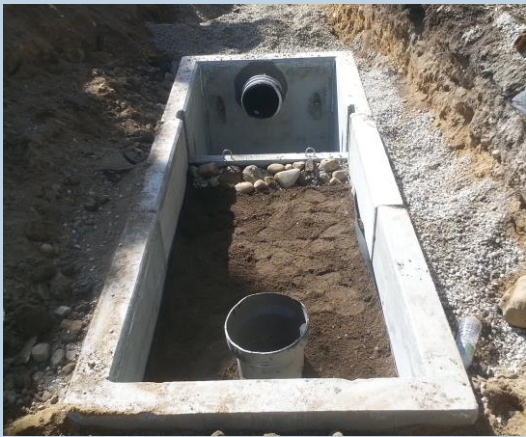
Photograph 8: Grove Street filtering catch basin.
