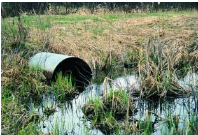
Wetland culverts allow for cross drainage if the road fill does not.
