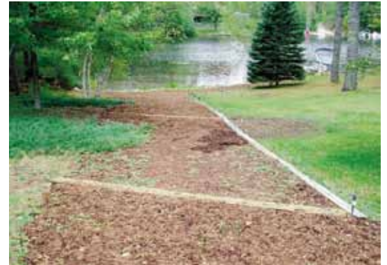
Waterbars along the path slow flow and divert runoff into the vegetated area.
