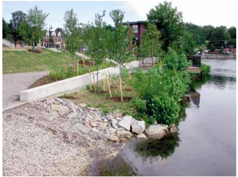
This 12-foot wide buffer is not adequate for the steeply-sloped property above it. The paved pathways provide a direct route for runoff water to enter the river.
