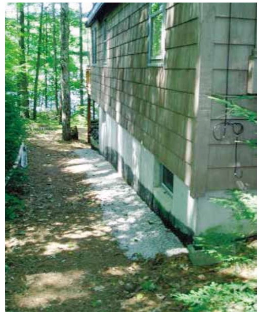
An infiltration trench was constructed to catch roof runoff at this lakeside home.
